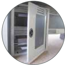
EQUIPMENT RACK (37107 IS)
