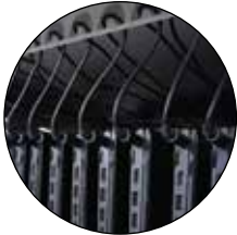
OVERHEAD WIRE MANAGEMENT
